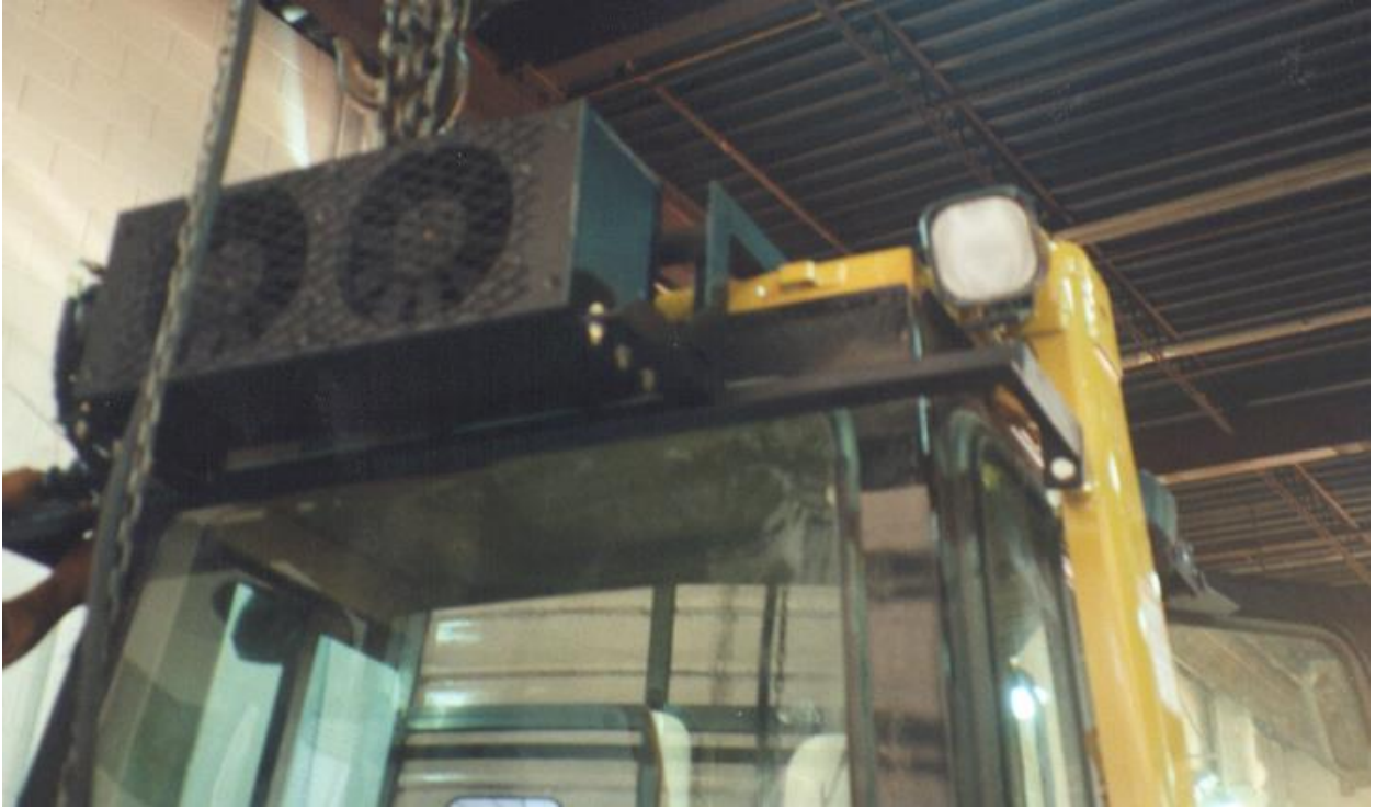
Right side of condenser assembly.
